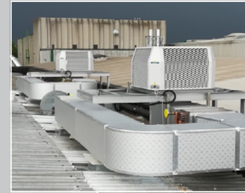
Waste treatment plant, Italy
